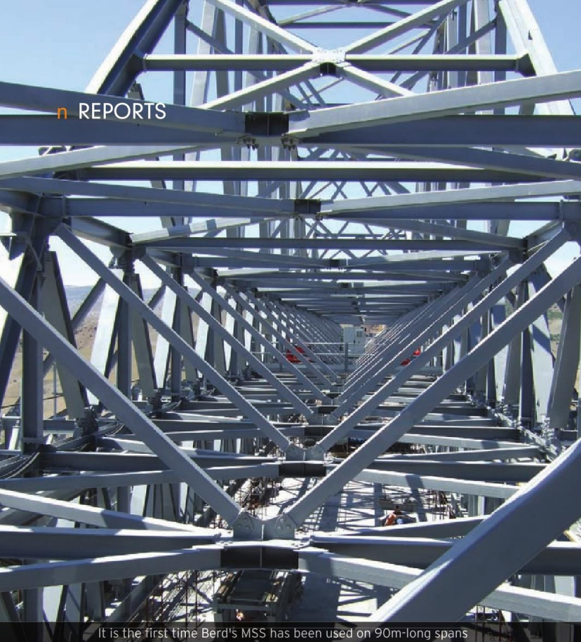
It is the first time Berd's MSS has been used on 90m-long spans
