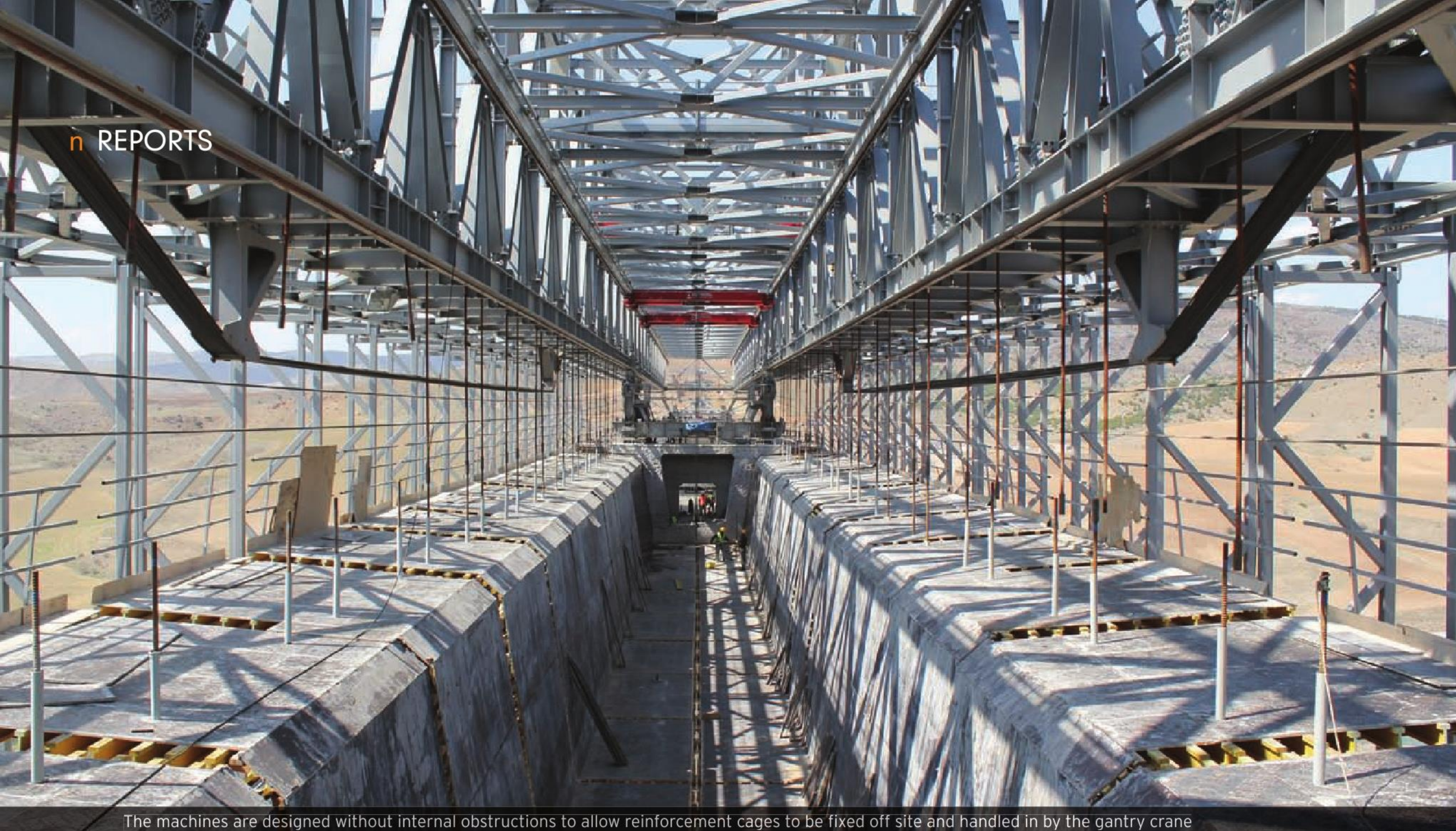
The machines are designed without internal obstructions to allow reinforcement cages to be fixed off site and handled in by the gantry crane
