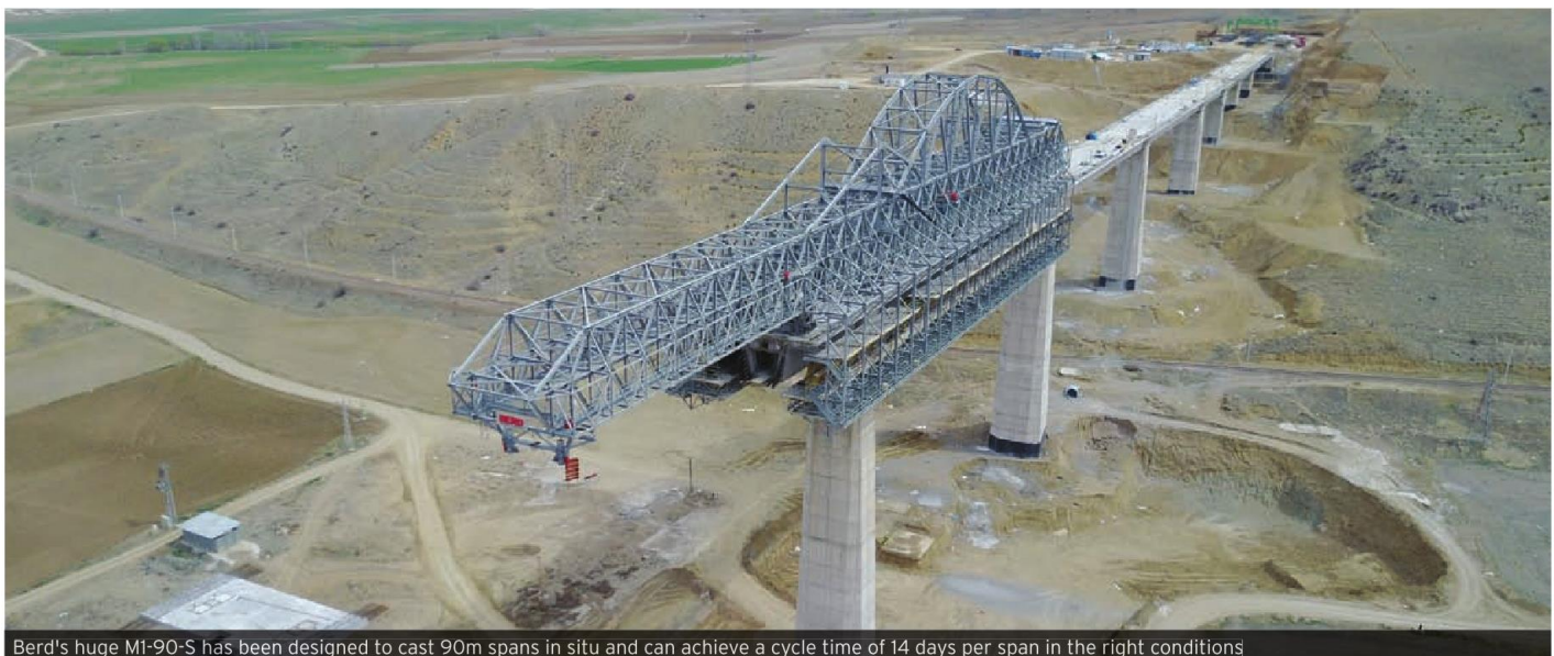
Berd's huge M1-90-S has been designed to cast 90m spans in situ and can achieve a cycle time of 14 days per span in the right conditions
